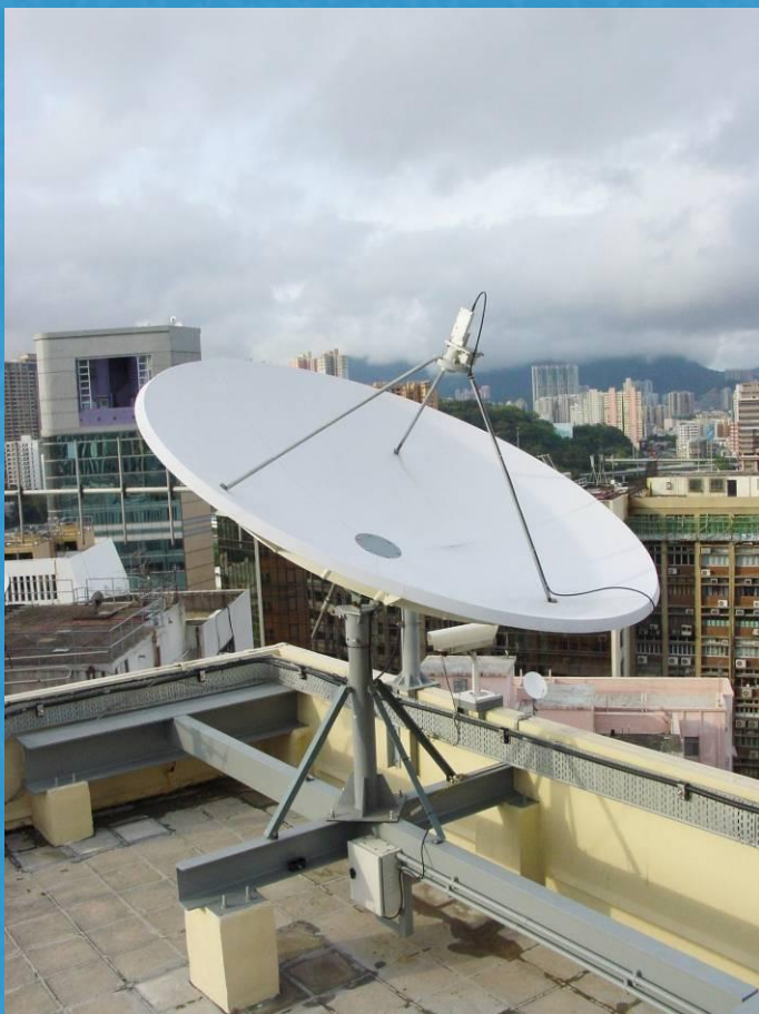
Reception antenna at HKO Headquarters
